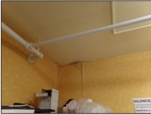
Peeling wall paper.
