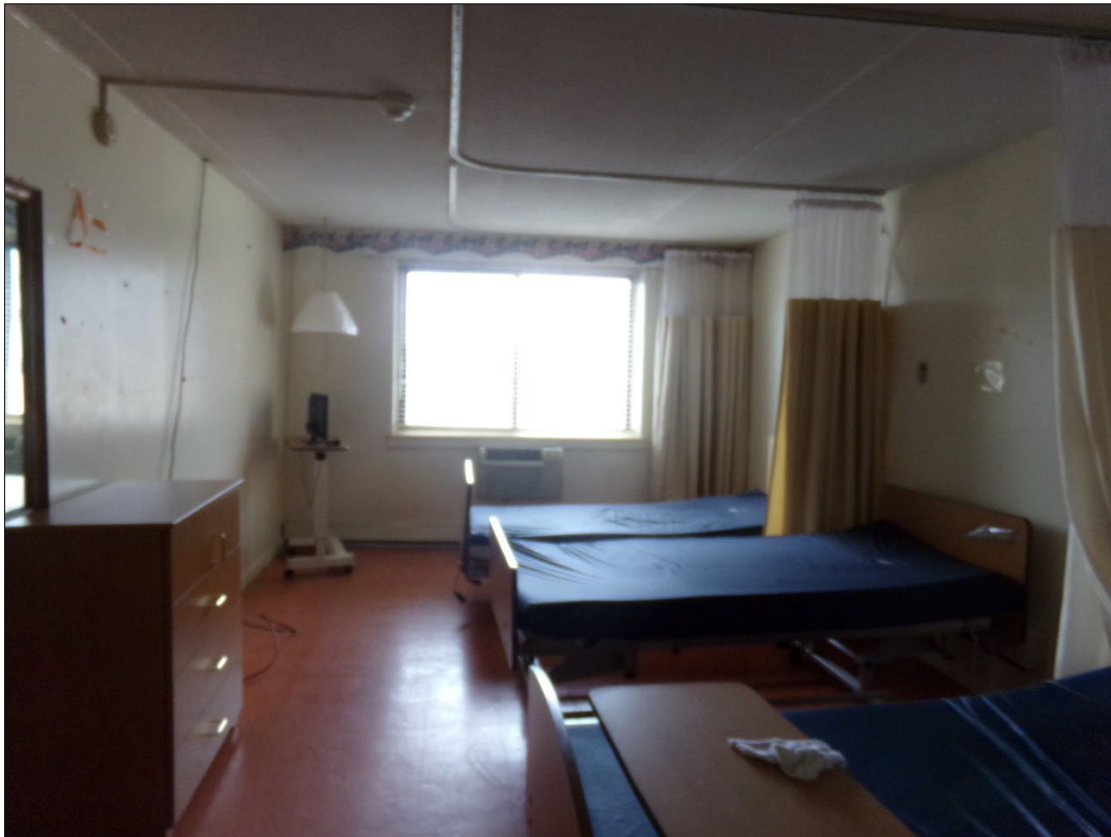
A.4 photos of rooms – CROWDING & DILAPIDATION
