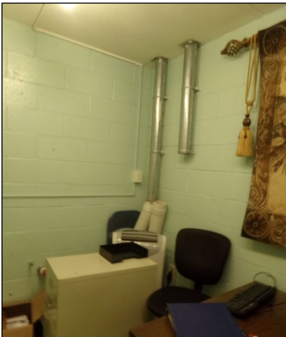
Exposed heating pipes.
