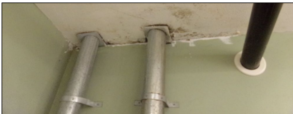
A.1 Improper Retrofitting
