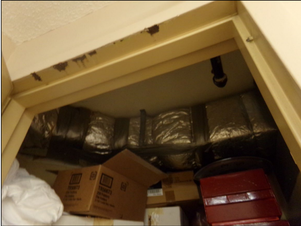
Exposed insulation in closets.
