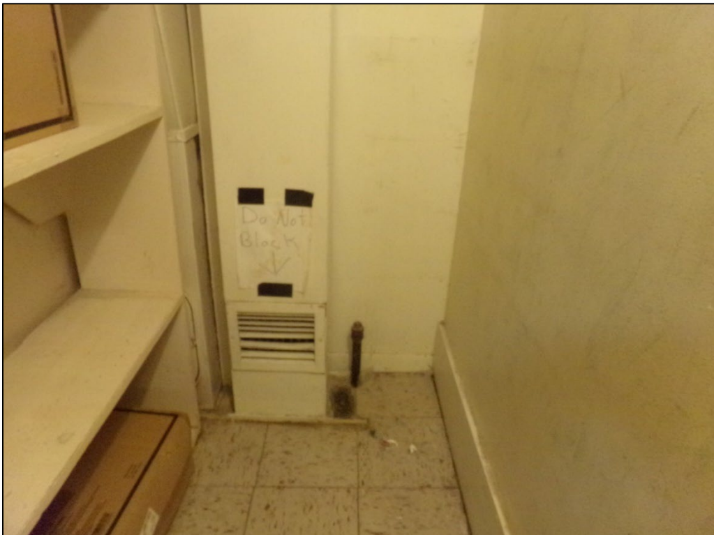
Small vents for HVAC.
