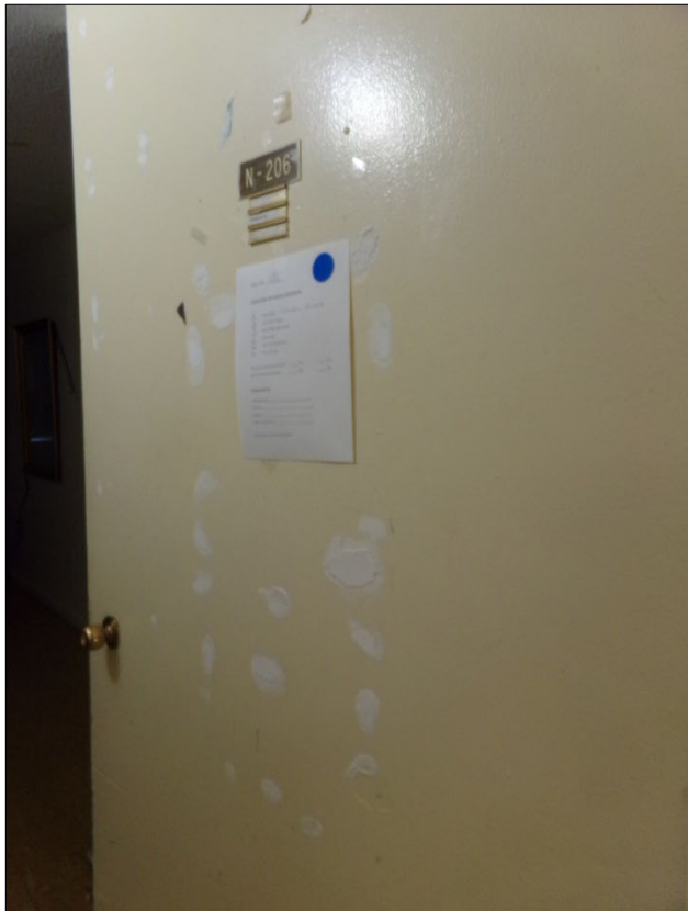
A.4 photos of rooms – CROWDING & DILAPIDATION
