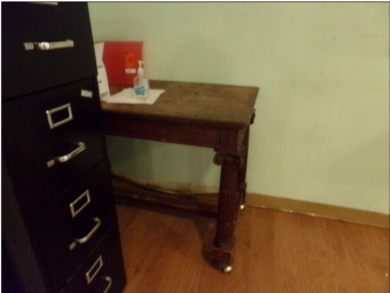
Peeling floorboard moldings.
